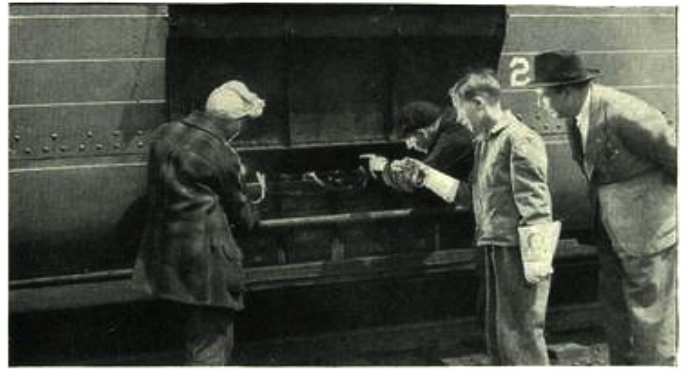
And here Jim holds the flashlight and his Dad watches while an electrician and his girl helper inspect the batteries under a passenger coach, to make sure that they are in perfect condition for the next trip. Air-conditioning, heating equipment and washroom facilities also are checked by other yard employees.
