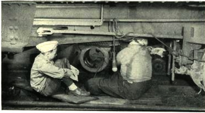
Jim was very much interested in watching electricians install a new generator under a passenger coach. The generator, which operates while the coach is running, keeps the batteries charged. The batteries, of course, supply the electricity for lighting the car—and also the power to run father's electric razor.
